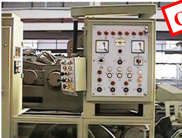
ORIGINAL OPERATING STATION
